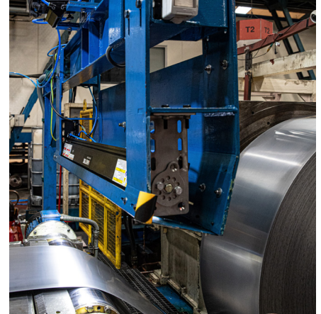
Figure 2 The SmartView® system installed on the skin pass mill
