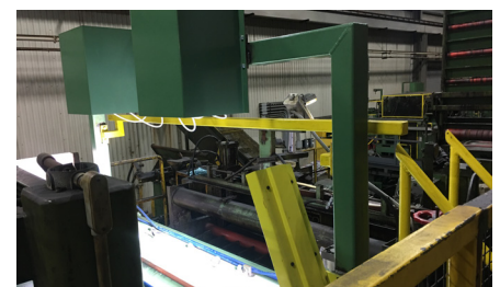
Installation of SmartView® surface inspection system at Samuel Nelson Steel, Stoney Creek, Ontario, Canada.
