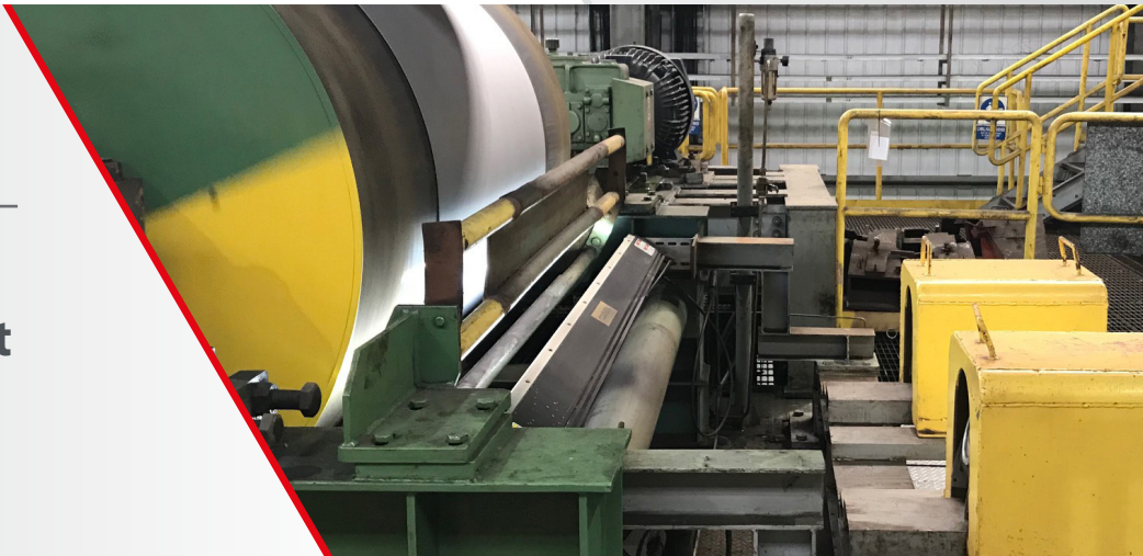
Figure 1: The SmartView system at the end of the pickling line in the Ternium Pesqueria steel plant
